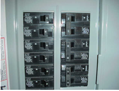
Circuit Breaker Box
